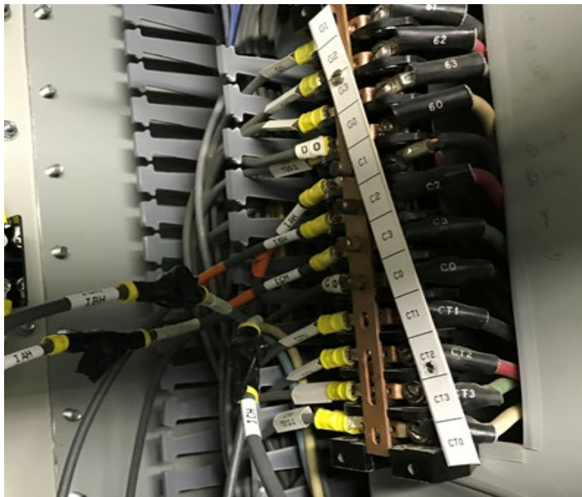
Photo 2 - CT Connection on Governor Cabinet
